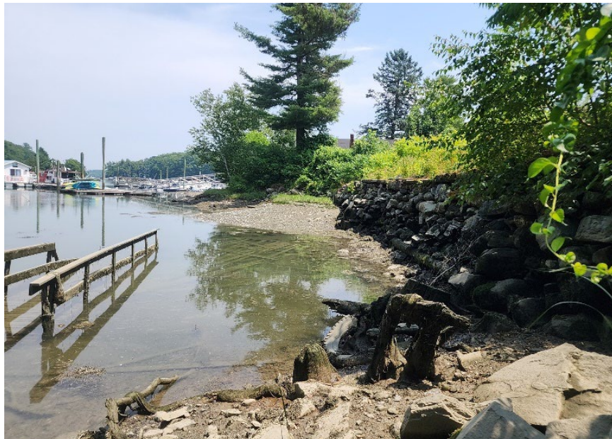
Photograph 5b: Looking south, view of cribbed stone retaining wall, from A-10 eastward (see Sheet 5); July 2024
